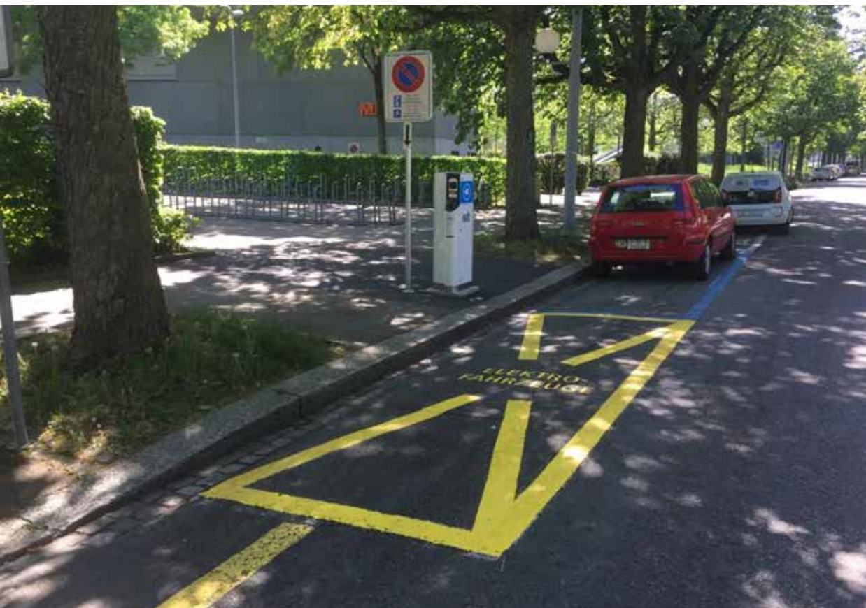
Quartierladestation in Basel
